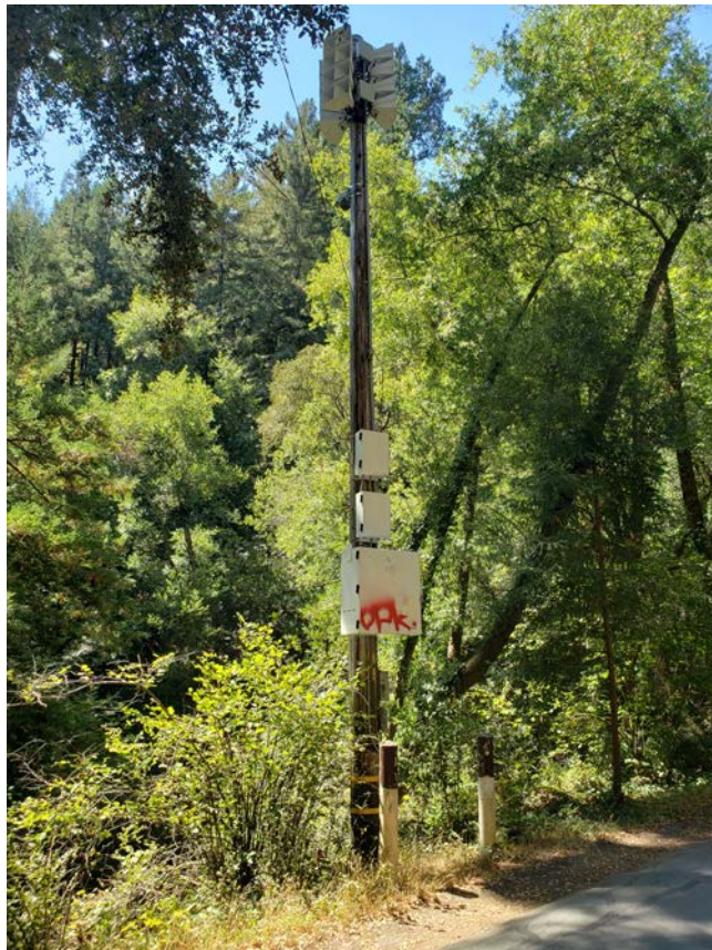
Figure 7 Example of LRAD Unit Installed Near Trees
