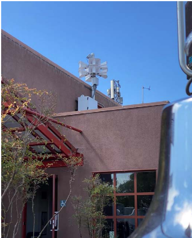
Figure 6 Example of LRAD Unit Mounted on a Fire Station
