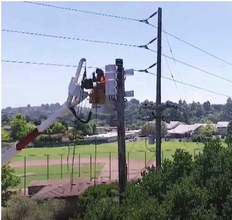
Figure 5 Example of LRAD Unit Installation Adjacent to Power Poles
