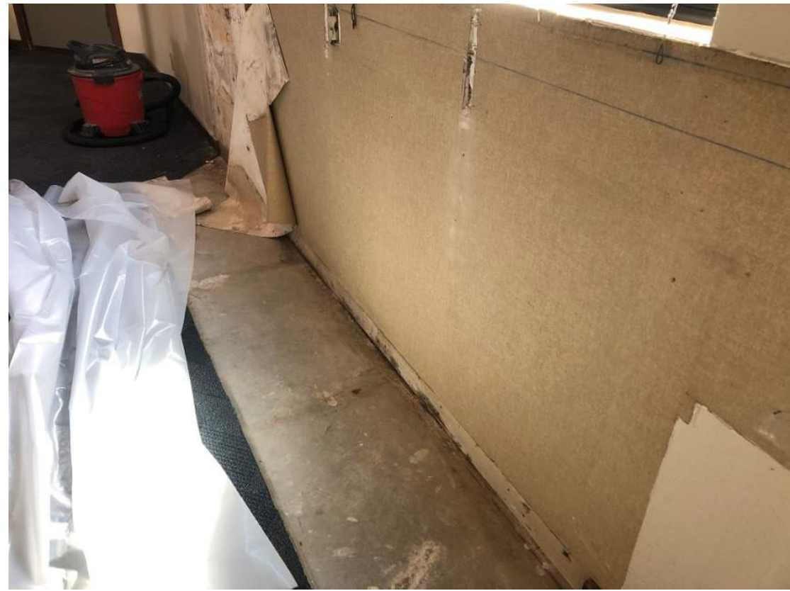
PHOTO 1 MOLD AT BASE OF WALL BELOW FIRE PREVENTION WINDOWS
