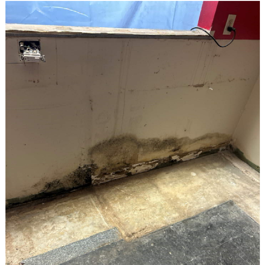
PHOTO 5: MOLD ON SURFACE OF WALL IN KITCHEN
